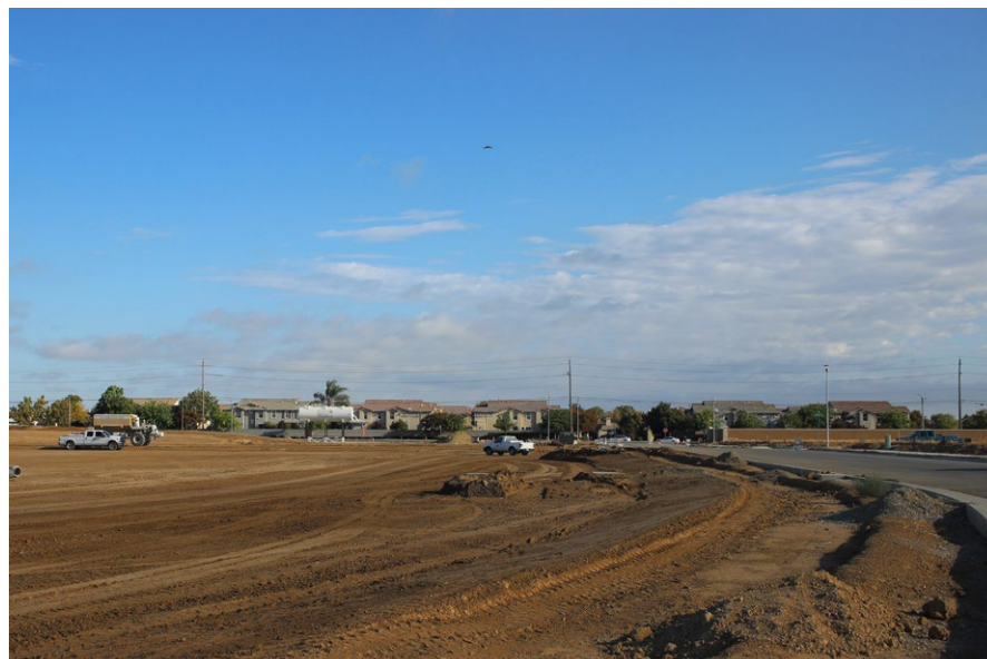
Figure 9. (Above) Sheldon Farms North Looking North from the Intersection of Mashpee Way and Barnstable Road
