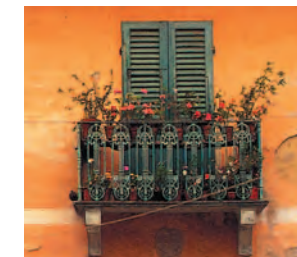
Wrought iron Juliet balcony with pre-cast supports
