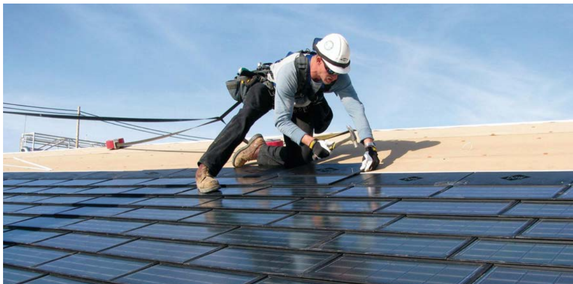
Integrated solar roof panels
