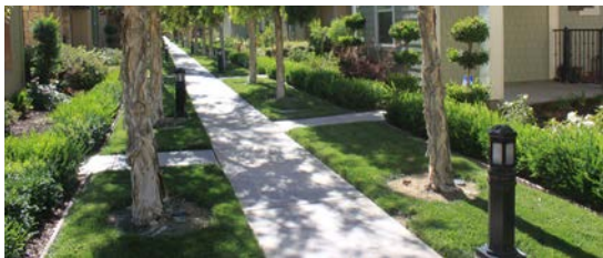
Exterior lighting along pedestrian pathway
