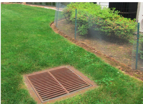
Figure 2. Dry well installed to receive runoff flowing through a lawn (Source: R. Pitt)
